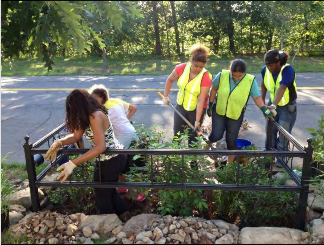
Figure X-XII. Homeowners and Common Ground High School students plant perennials in a New Haven Bioswale
